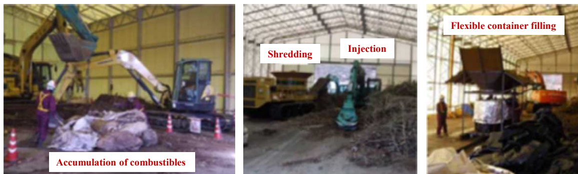
Figure 3-17 Interior views of a crushing facility: collection (left), putting in and crushing (center), and packing into flexible containers (right).
