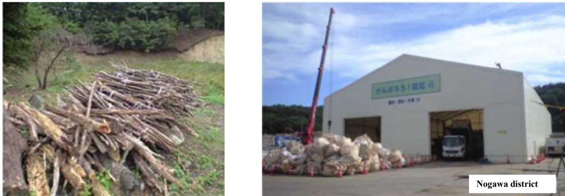
Figure 3-16 Branches cut down (left) in forest decontamination and a crushing facility (right) 89 .
