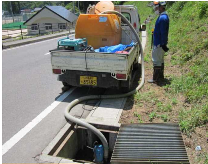
Figure 3-12 Treatment of wastewater used in washing (Kawauchi Village) 84
